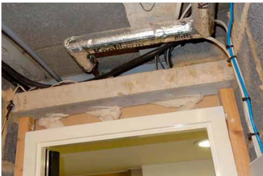
2016 - The contractor, building control officer and fire risk assessor all thought this services’ riser fire door was okay...
