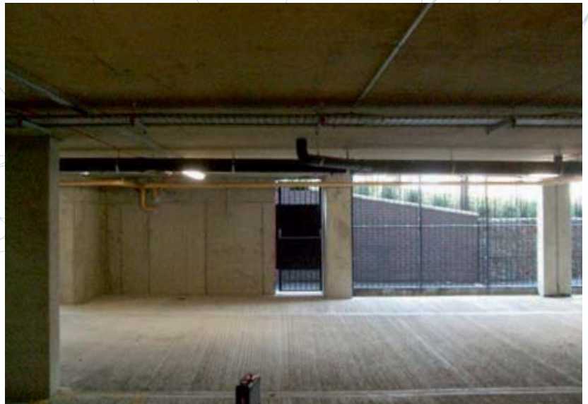
A brand new car park below a multi-storey building opened in 2013. Spot the fire exit sign? It’s behind the gas pipe. Signed off by the Building Control body but the construction delivery team remains liable for this defect
